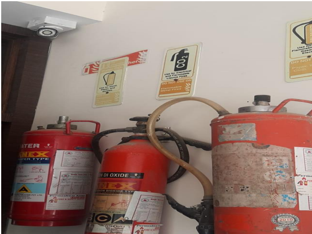
Fully equipped Fire extinguisher
